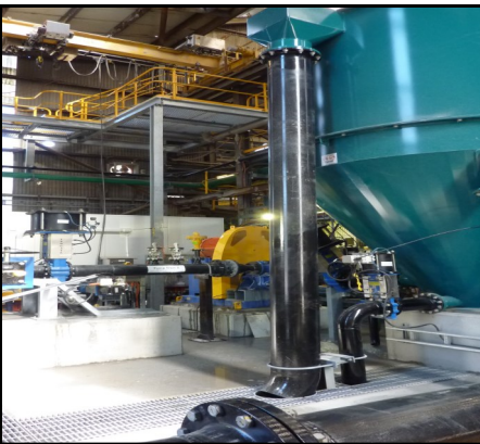
Pump station with slurry tank, pipe work and supports, switchroom and crane maintenance platform
