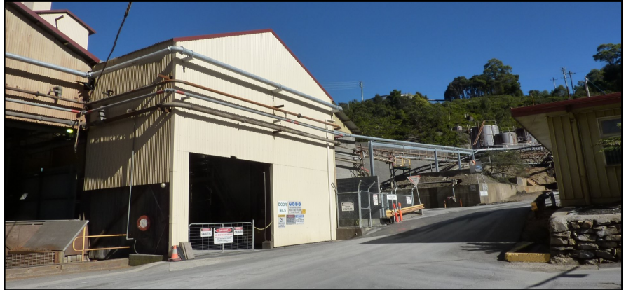
Pipe bridge across road and steel pipe with pipe supports on building
