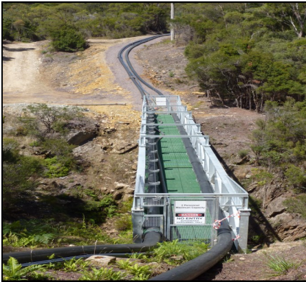
HDPE pipe across Stitt River Bridge
